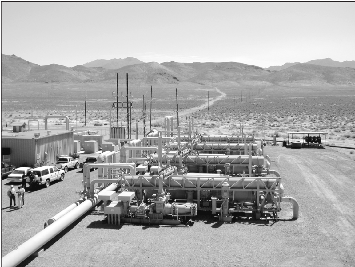
Binary generation units at the Empire Farms geothermal plant and garlic and onion drying facility. Photo by Larry Garside, 2001.
